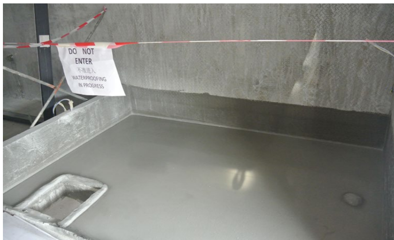
Waterproofing membrane at wet areas
