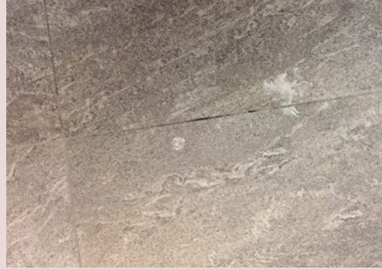
Paint stains Figure 5.5.f
