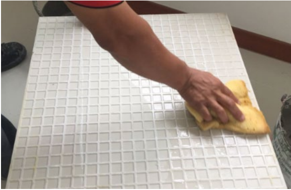
Cleaning ceramic tile to remove dirt and dust before laying Figure 5.2.a
