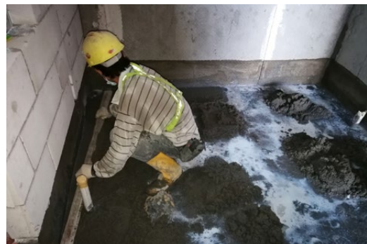
Levelling the screed to a flat surface with timber/aluminum trowel Figure 4.2.1.d
